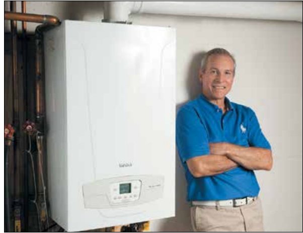
Homeowner Bobby Brown of Port Washington, N.Y. says house guests marvel at his sleek-looking, quiet and highly efficient Baxi wall-hung boiler, installed by SAC plumbing and heating. The gas-fired Baxi combination heating and domestic hot water has improved home comfort significantly — freeing up valuable living space, cutting greenhouse gas emissions, and reducing the homeowner's energy bills by over 70 percent versus his former oil heat. (Baxi systems in retrofits typically cut utility costs from 35 to 70 percent.)
